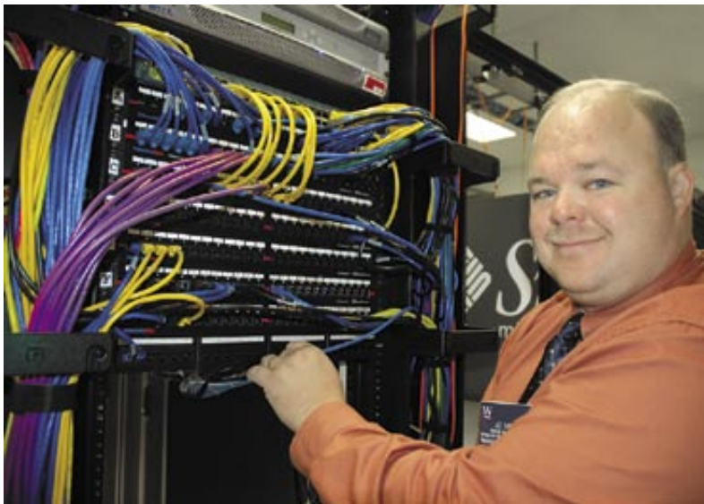
Joe Sargent, director of communications services at WSCC, inspects one of the wiring closets serving the school's varied network.
